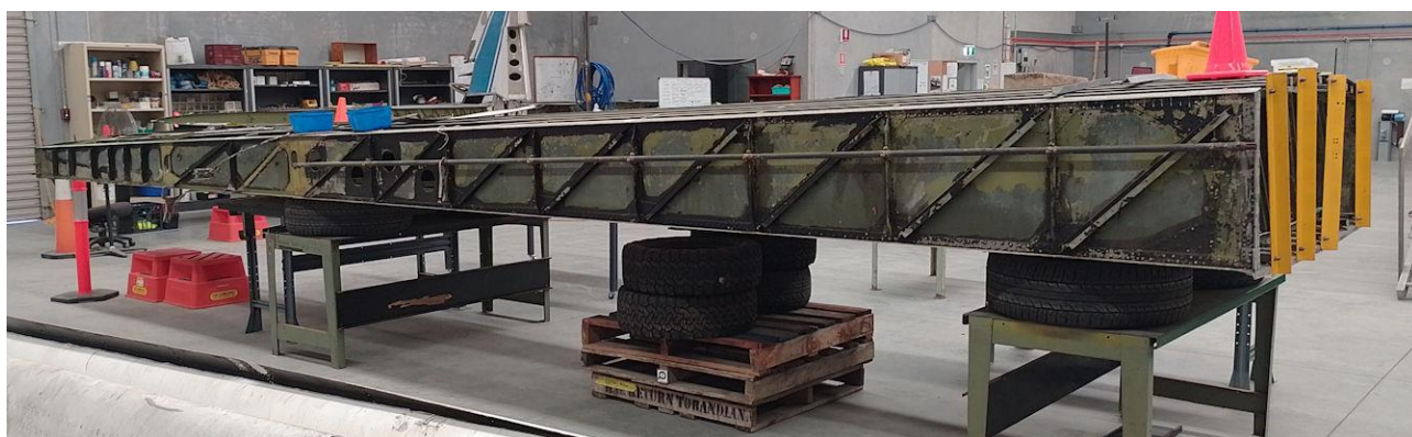
Above is the end wing with the outside skinned removed. They must repair all the corrosion inside, before reattaching the outer skin. Below, the back section is completed and has been painted in grey.
